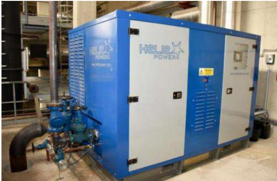
Figure 21: Helix GenSet installation in Obertrum am See (A) [15]
