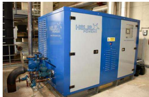
Figure 20. Heliex GenSet installation in Obertrum am See (A) [59].
