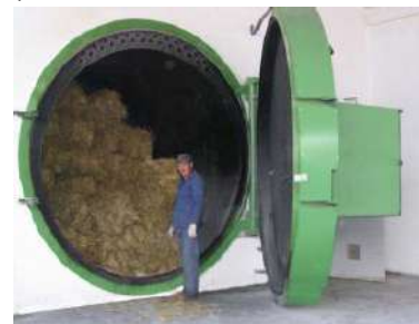
c) biomass boiler
